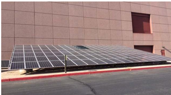
Figure 1. The SenSIP 18kw (104 panel) experimental facility established at ASU with industry collaborators.
